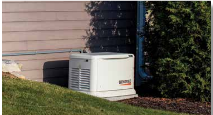
Photo & article compliments of Generac.
